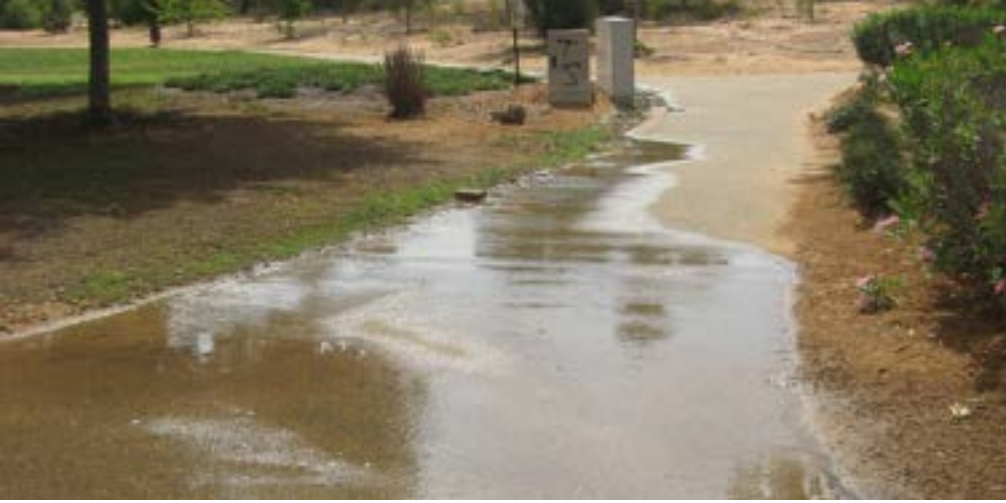
Image 2 - Water logging due to an inadequate design and/or operation of the irrigation system in a slope area. Photo: Avigail Heller
